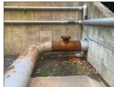
Figure 27: Exterior water tower with signs of degradation including a replacement of a section of the pipe due to failure
