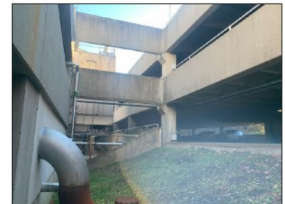
Figure 30: Exterior water tower with signs of degradation including a replacement of a section of the pipe due to failure
