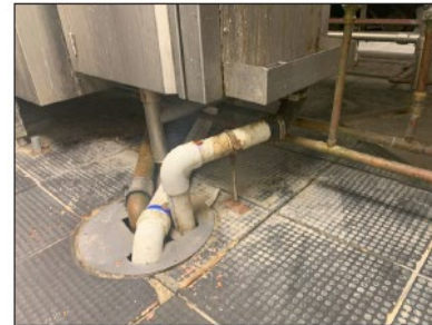
Figure 45: Kitchen washing area with replaced pipes do to failure
