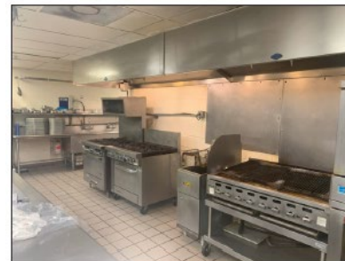
Figure 47: Existing kitchen with original equipment in need of replacement.
