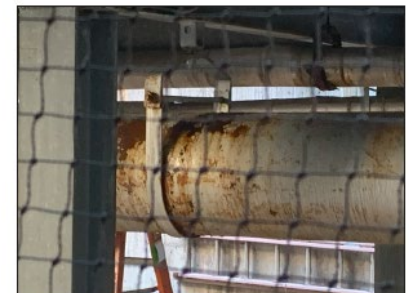
Figure 28: Exterior water tower with signs of degradation including a replacement of a section of the pipe due to failure
