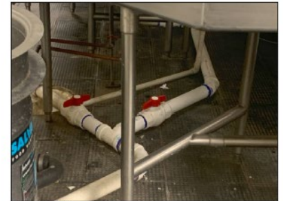
Figure 46: Kitchen washing area with replaced pipes do to failure
