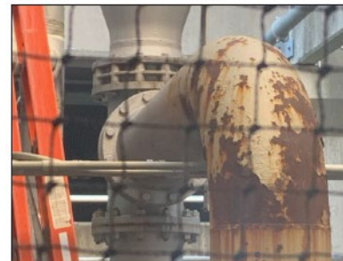
Figure 29: Exterior water tower with signs of degradation including a replacement of a section of the pipe due to failure
