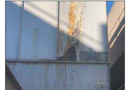
Figure 26: Exterior water tower with signs of degradation
